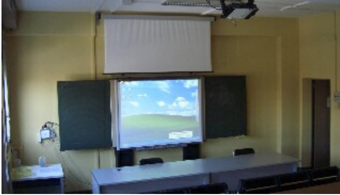
Fig. 4. A typical digital whiteboard installation: note the presence of the traditional blackboard and the installation of the PC fixed to the wall on the left
